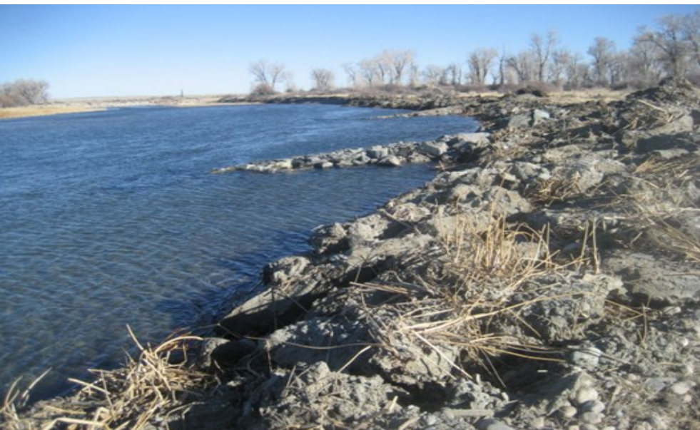
Freshly completed bank stabilization features on the Green River at Lunch Island.
