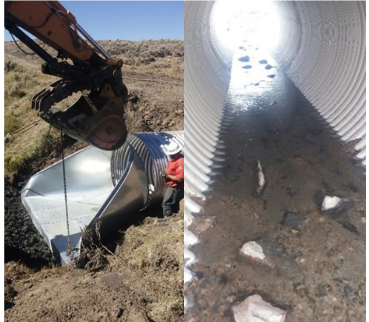
Littlefield Creek culvert installation. The culvert was bedded with cobble and gravel to improve fish passage and stream stability.
