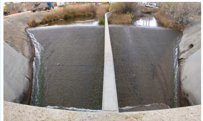
Figure 2. The 12 foot concrete ramp located just upstream of Interstate 25 on Clear Creek in Buffalo, WY. The removal of the ramp will allow fish movement throughout Clear Creek.
