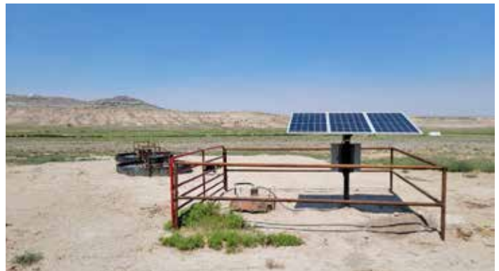
Twin Peaks well new solar array and two tire tanks.
