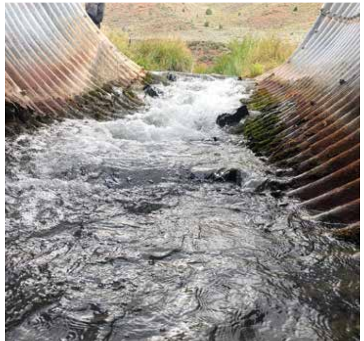
Baffles slow water and increase depth within a culvert inlet.
