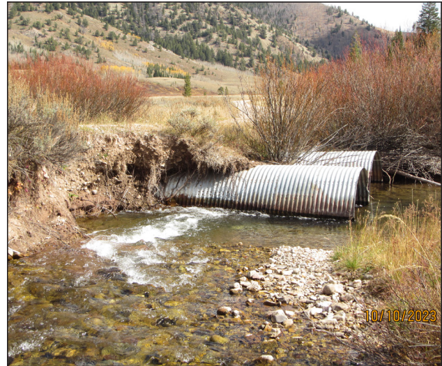
Figure 2. A surveyed crossing with undersized culverts.
