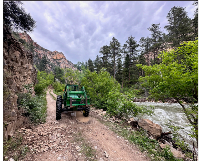
Figure 152. Rock slide removal at Tongue River PAA.
