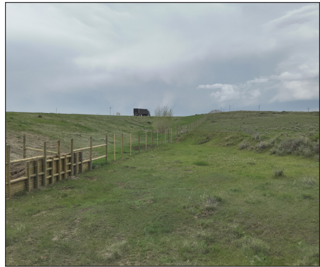
Figure 8. Wildlife-proof fence constructed along I-25 to reduce wildlife-vehicle collisions.
