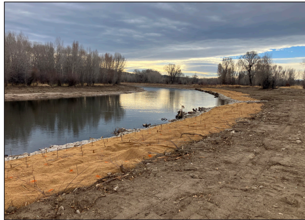
Figure 104. Restoration with toewood and bankfull benches with willow plantings on the North Platte River.
