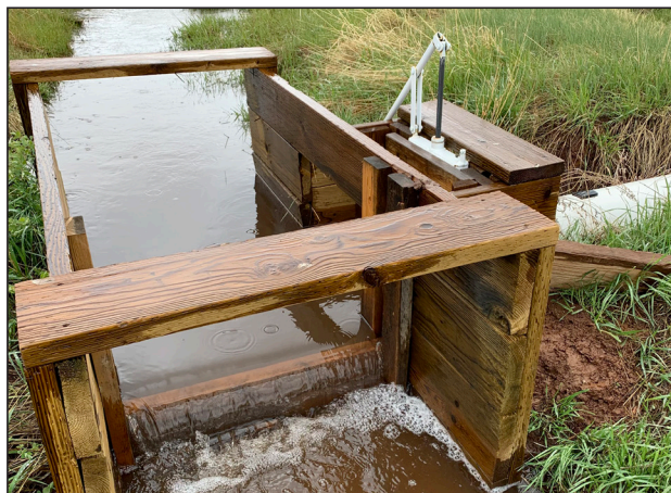
Figure 92. New irrigation diversion box on Wick WHMA.
