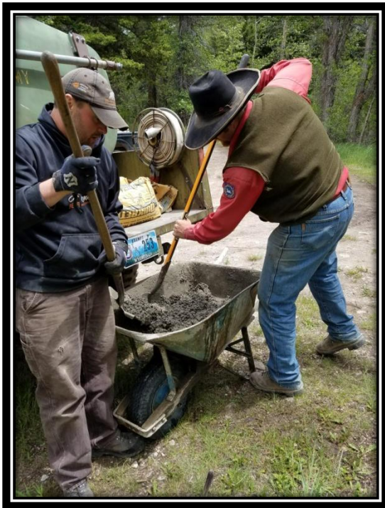
Joe Kondelis from Western Bear Foundation and Miles Proctor from the Department's Habitat and Access Branch mix cement to place a bear box.
