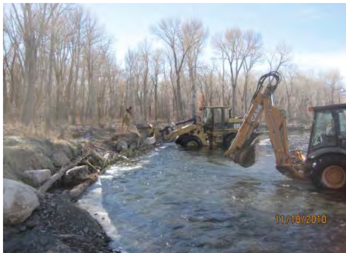
Figure 7. Rocks were used in combination with cable to hold trees in place to increase woody debris for fish habitat.
