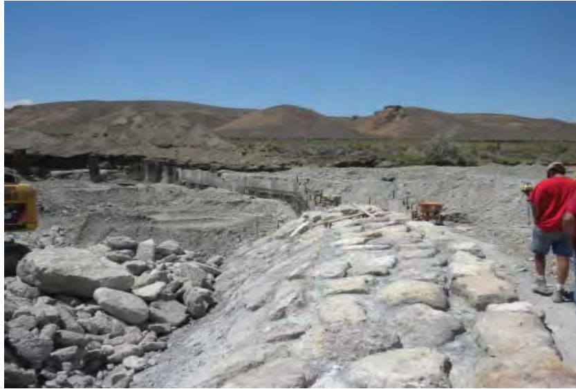
Figure 22. Installation of sill in the Green River. The sill will aid in watering the Killdeer Wetlands.
