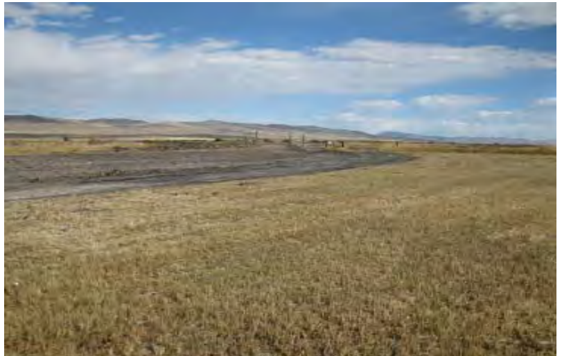
Figure 21. Example of the repairs made to the BQ Dike to prevent water in the dike returning to the Bear River.
