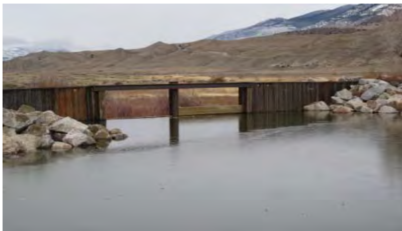
Figure 26. New water level control structure installed to create a wetland and silt detention pond to protect the Diamond Creek Dike Pond.
