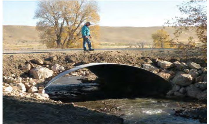
Figure 3. Timber Creek bottomless arch culvert installed in 2010 to provide fish passage, better stream dynamics, and prevent road flooding.
