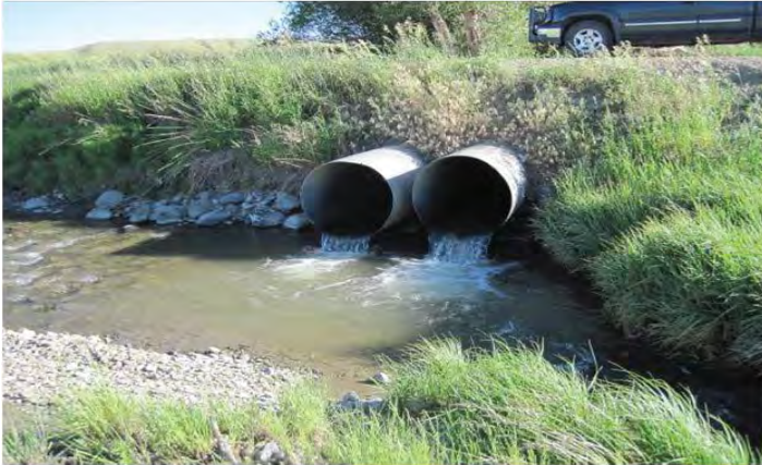
Figure 2. Timber Creek road crossing culverts replaced in 2010 to eliminate a barrier to Yellowstone cutthroat trout.
