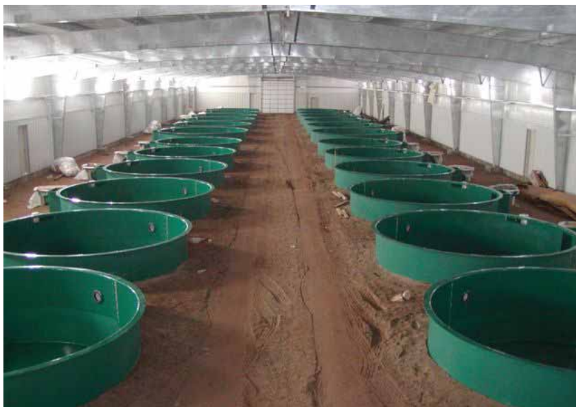
Fiberglass Rearing Units, there are now 12-foot, 16-foot and 20-foot circulars at Speas for a total of 36 new rearing units.
