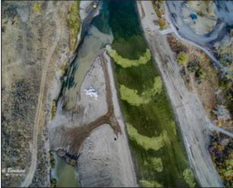
Figure 16. Construction on the North Platte Morad Park Site showing a construction crew narrowing the channel and creating a wetland. White half moon shapes in the river are partially constructed rock riffles.
