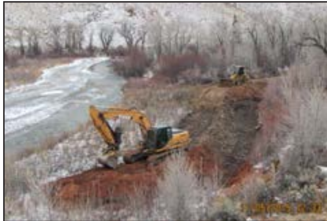
Figure 4. Excavation of the East Fork Ditch near the new diversion location on the East Fork Wind River.
