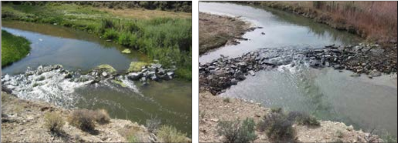
Figure 55. Before (left) and after (right) maintenance improvements to Sill “D” on the lower Big Sandy River.
