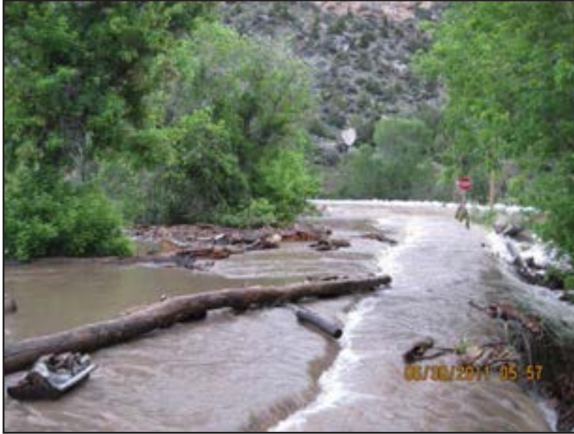
Figure 31. Flooding and debris jams at culverts three hours prior to the road washing out on June 30, 2011.
