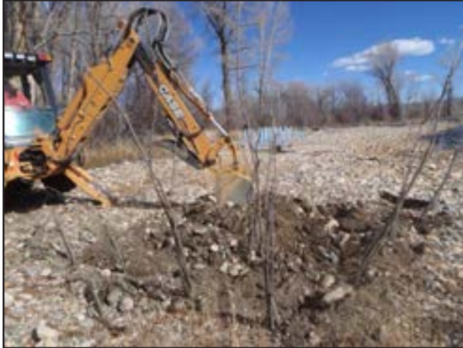
Figure 101. Digging holes and planting live stakes for the Encampment River “deposition and recruitment” plots.
