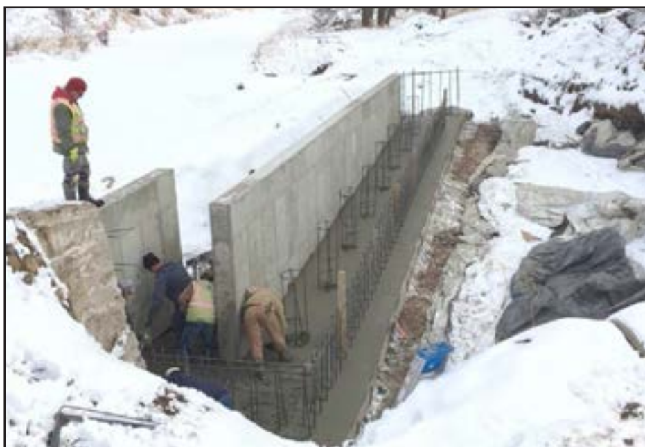
Figure 157. Construction of a fish ladder at the Pratt and Ferris #1 diversion dam on Piney Creek.
