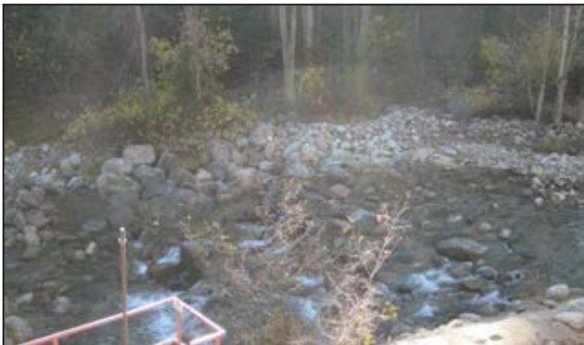
Figure 153. Graded rock patch to temporarily stabilize the toe of the Mead Coffeen Crossover Diversion grouted riprap dam.
