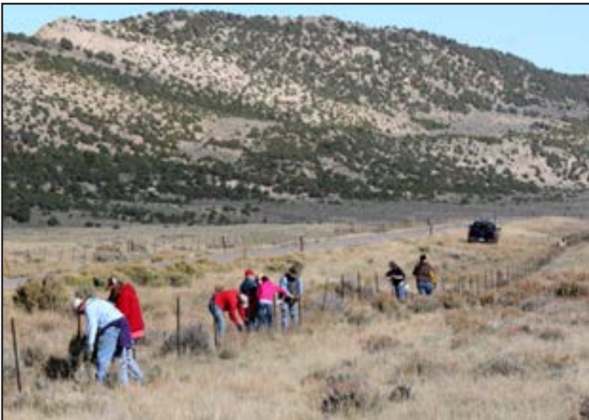
Figure 47. Students from the Youth Alternative School in Kemmerer remove unnecessary net wire fence along the sulfur haul road.
