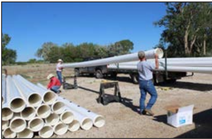
Figure 39. Around 600 linear feet of gated pipe was purchased for the project.
