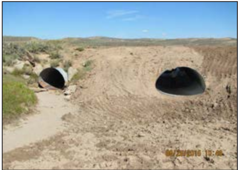
Figure 5. Looking downstream, the new culvert on the right doubles the flow capacity of the road crossing.
