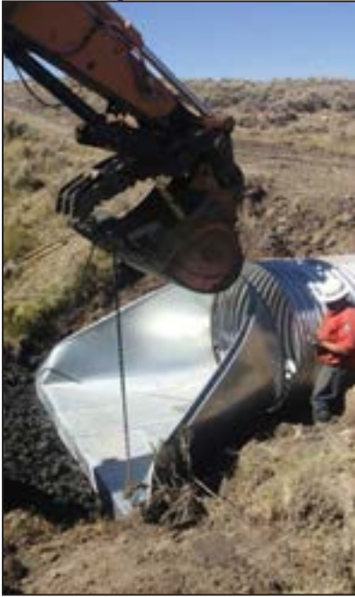
Figure 69. Statewide Habitat and Access crew replaces Littlefield Creek culvert at Grizzly WHMA.
