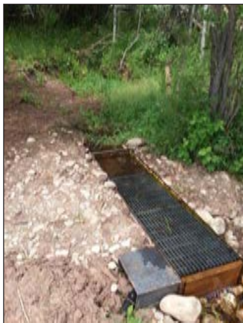
Figure 149. Spring intake box.
