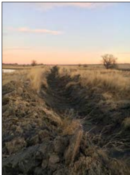
Figure 141. Bump Sullivan ditch after maintenance.
