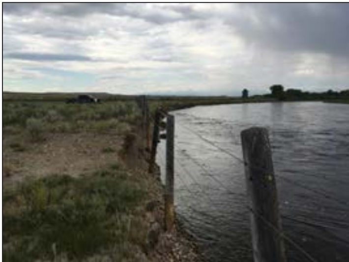
Figure 176. Eroding fenceline on the New Fork River on the property of a private landowner. Working with this landowner, this restoration will address sedimentation from a bank that is approximately six feet high and 1600 feet long and laterally migrated up two feet annually.
