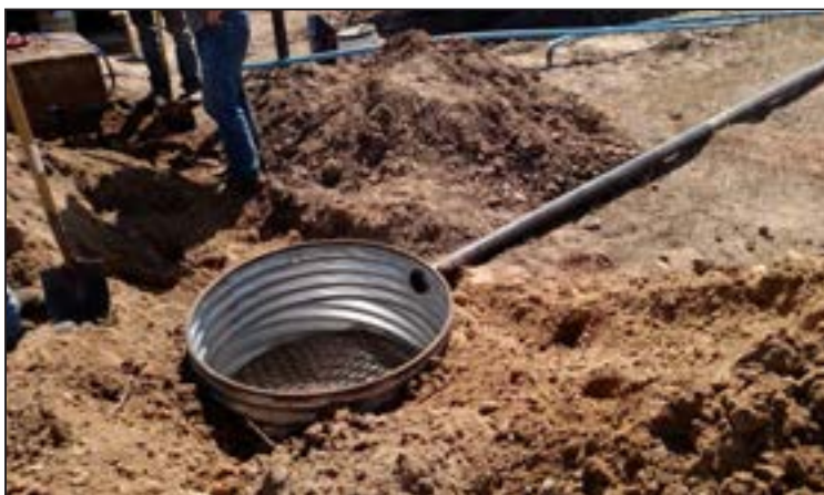
Figure 26. New culvert tank installed in bighorn sheep winter range on Elk Mountain.
