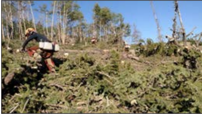
Figure 205. Contract crew removing conifers from an aspen stand in the head of the Tongue River Canyon.
