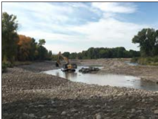
Figure 132. Constructing rock barb in “the dry” while flows are bypassed around construction area at North Platte River - Ryan Ranch Restoration Phase 2.
