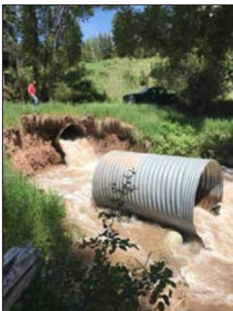
Figure 98. Horse Creek irrigation diversion failure and road loss, June 2017.
