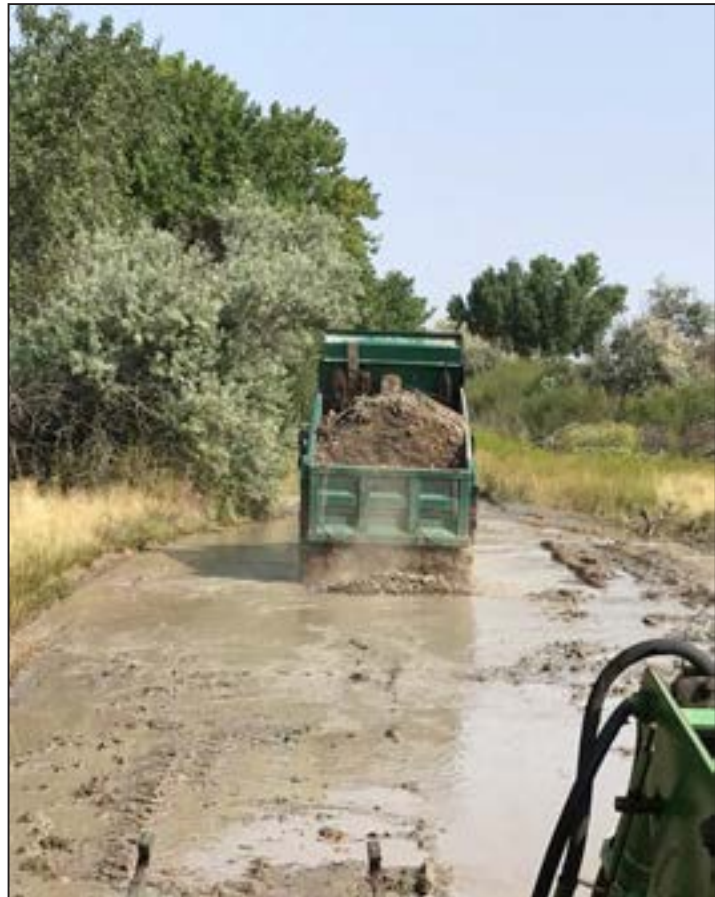
Figure 40. Gravel being dumped in a large sink hole on a Yellowtail WHMA road.
