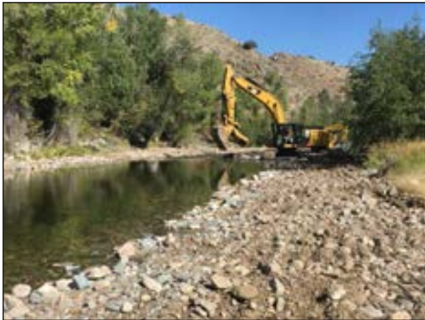
Figure 146. Constructing boulder clusters in narrowed, deepened channel at the Encampment River - Oddfellows Phase 2 site.
