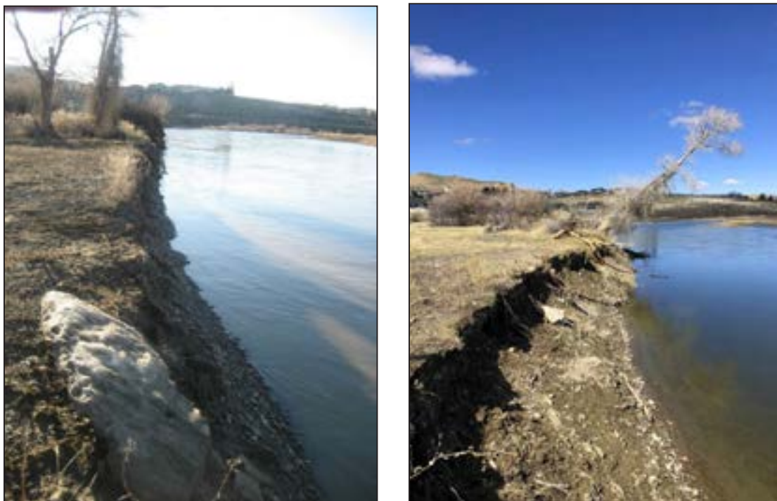
Figure 78. Photo point along the Green River at Scott's Bottom comparing bank erosion between 2017 (left) and 2018 (right).
