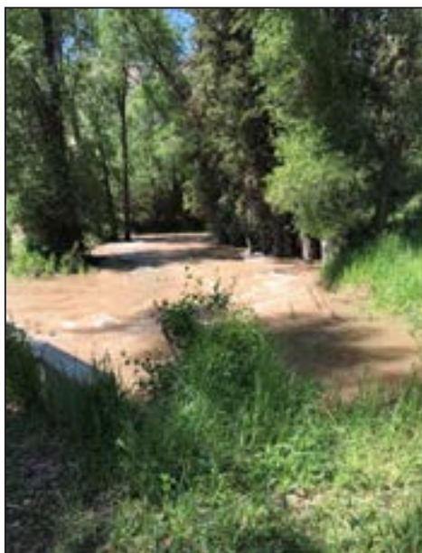
Figure 99. An upstream view of the Horse Creek irrigation diversion in 2017 shows significant backwater ponding upstream of the undersized culvert.
