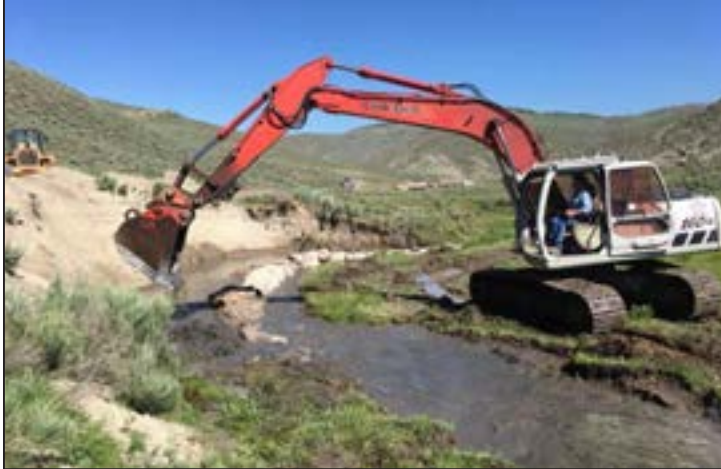
Figure 184. Excavators build a bankfull bench on Coal Creek to reduce erosion from the raw, vertical bank.
