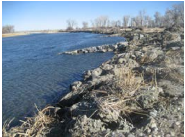
Figure 71. Freshly completed bank stabilization features on the Green River at Lunch Island.
