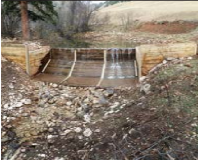
Figure 199. A timber crib barrier constructed on the North Fork of West Pass Creek secured 1.7 stream miles of habitat for native YSC.
