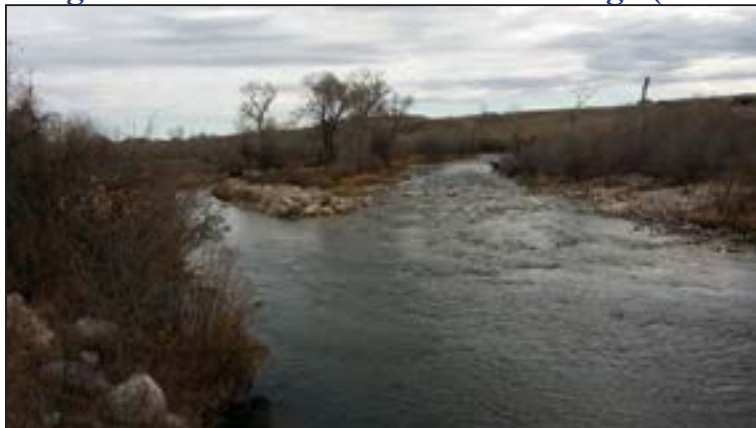
Figure 196. New ramped vane structure completed at the Tongue River #1 Diversion (also known as the Green Ditch) on the Tongue River.
