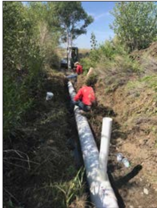
Figure 37. Habitat and access personnel install transport pipe to the 30 acre permanent cover field.
