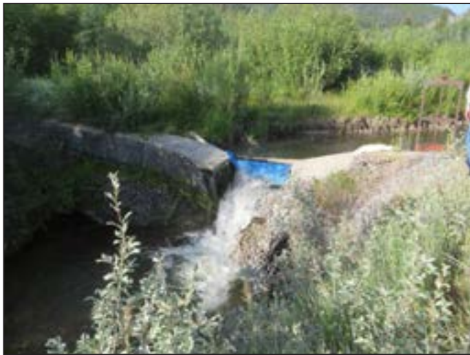
Figure 4. Dick Creek diversion gabion baskets are close to failure.
