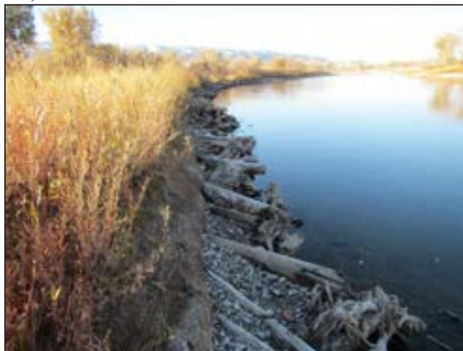
Figure 29. A toe wood structure constructed along a bend in the Wyoming Boulevard restoration site protects the bank from erosion and provides cover for trout. Willows have established well above the structure and will improve long-term bank stability.
