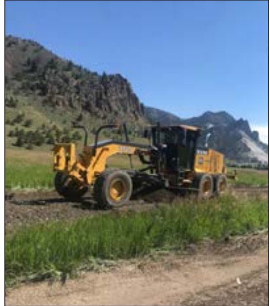
Figure 58. Habitat and Access personnel use a motor grader to repair Sunlight WHMA roads.
