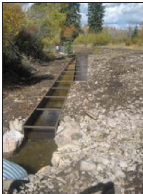
Figure 82. Farmer's Conservation Alliance flat plate fish screen installed at in irrigation diversion in the upper Bear River.
