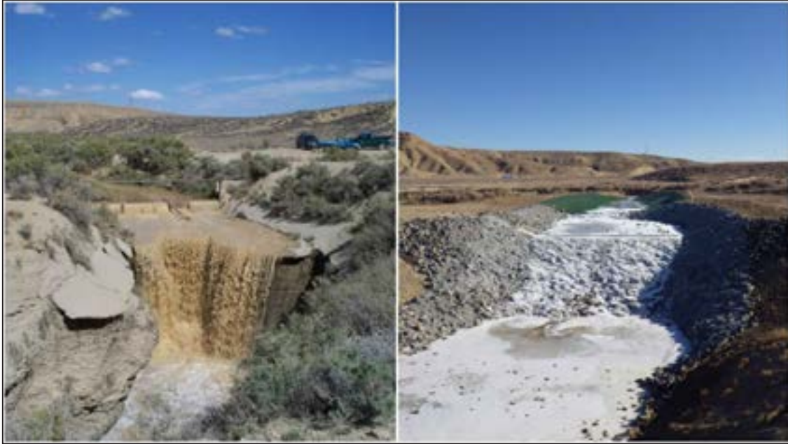
Figure 72. Before and after photos of the Bitter Creek drop structure. Photo courtesy of Sweetwater County Conservation District.
