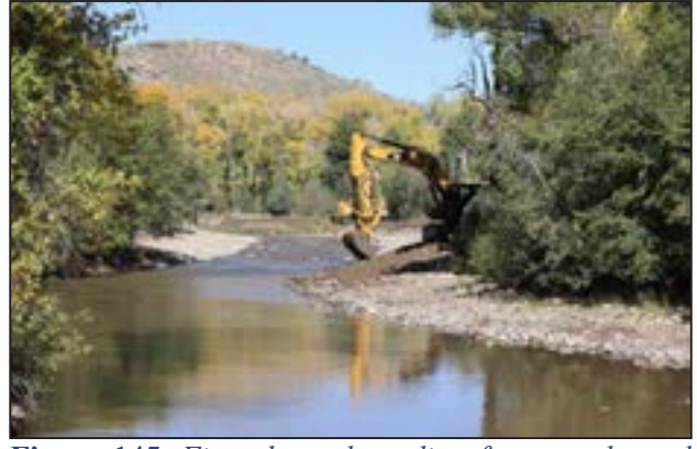
Figure 145. Fine channel grading for new channel dimensions on the Encampment River Pickett Restoration.
