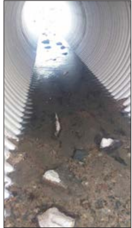
Figure 70. New Littlefield Creek culvert bedded with cobble and gravel to improve fish passage and stream stability.
