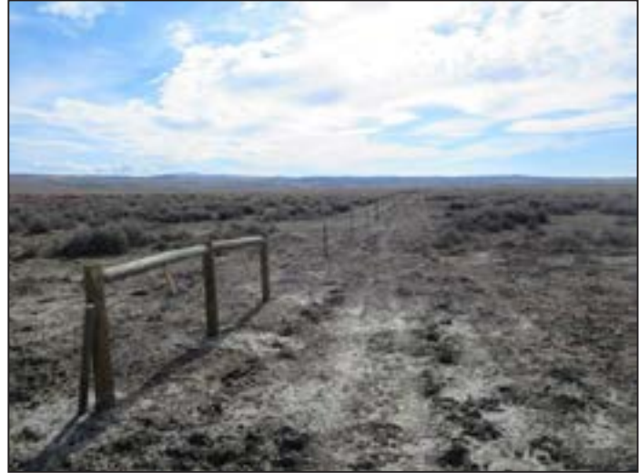
Figure 112. New fence on the Red Rim - Daley constructed to make the Shipping Pasture more user-friendly.
