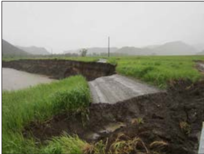
Figure 57. Road washout on Sunlight WHMA.
