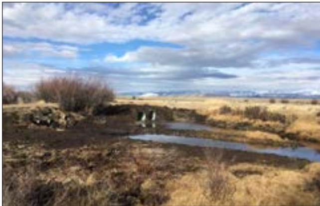
Figure 157. Road culvert addition and repairs at Airport Access on the New Fork River.
