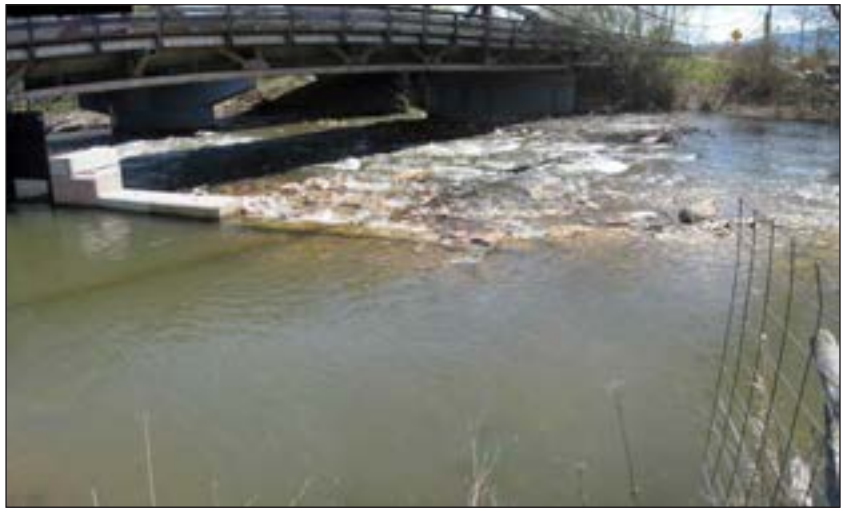
Figure 165. New sluiceway liftgate (upper left of photo) at the Hanover Diversion structure on the Tongue River.
