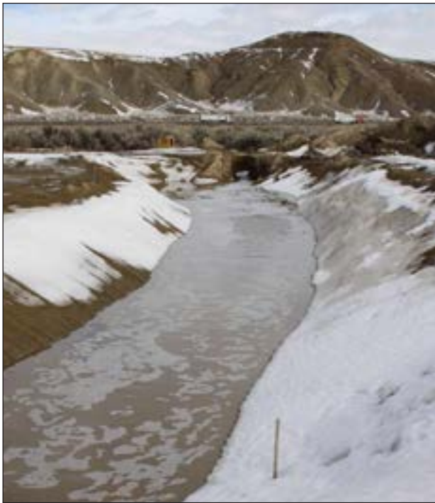
Figure 56. Bitter Creek Diversion Ditch conveying high water impacting the construction site. Photo credit Sweetwater County Conservation District.
