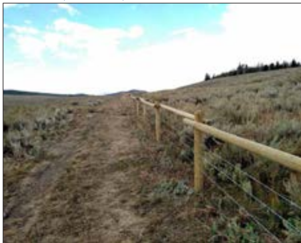
Figure 126. Newly constructed fence on the Rim Ranch is intended to decrease wildlife fence-related mortalities.
