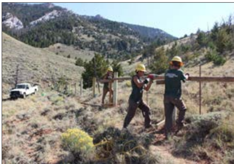
Figure 91. Montana Conservation Corps crew modifying old barbed wire and mesh wire fence to wood post, rail-top and wire fence at Ferris Mountain. Photo credit BLM.
