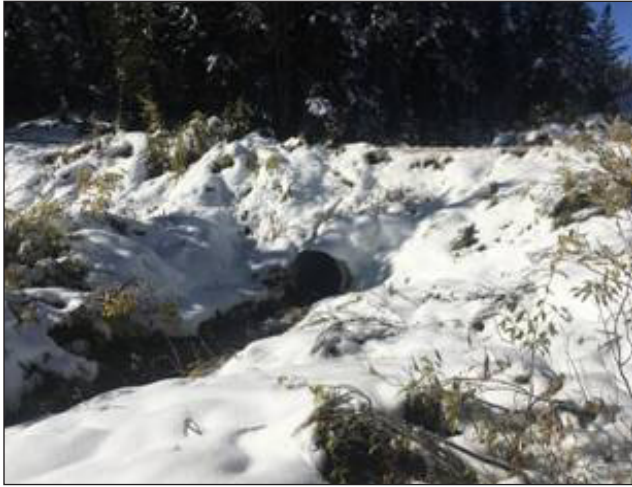
Figure 1. Crystal Creek before replacement of undersized culvert.
