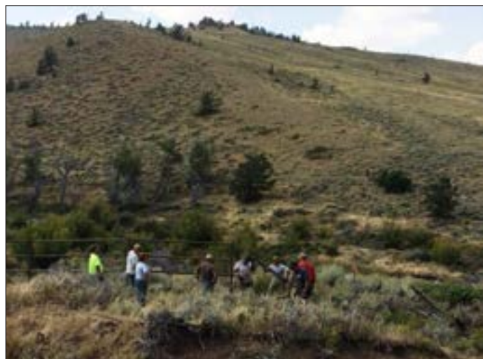
Figure 94. Construction of drill stem pipe fencing around an important riparian wetland located on West Cottonwood Creek, Green Mountain.
