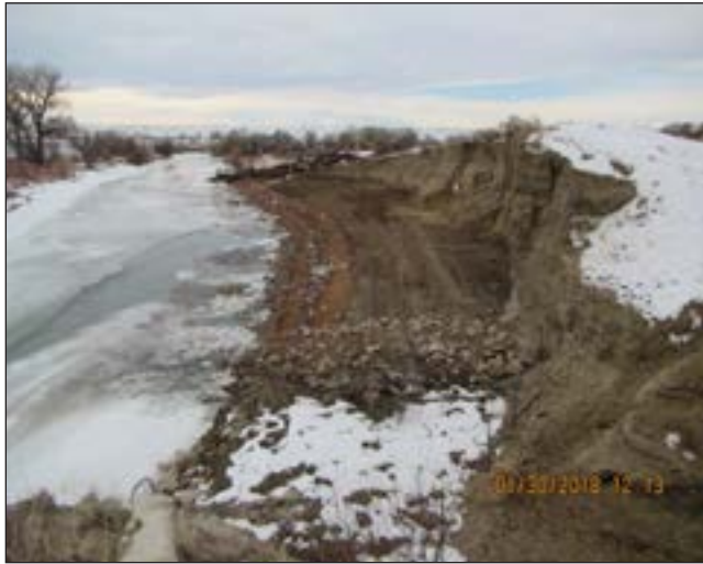
Figure 10. Toewood/bankfull bench to stabilize a highly erodible terrace and stabilize the river upstream of the POD.
