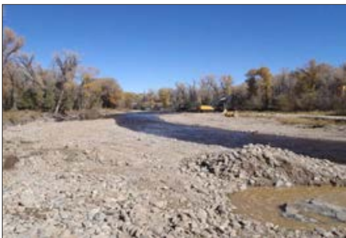
Figure 112. Constructing a narrower and deeper channel at the Encampment River-Riverside Phase I Restoration.
