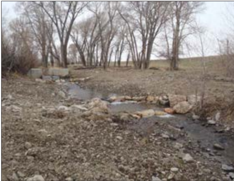
Figure 9. Cross vanes installed downstream of a concrete box diversion structure assist with upstream fish passage.
