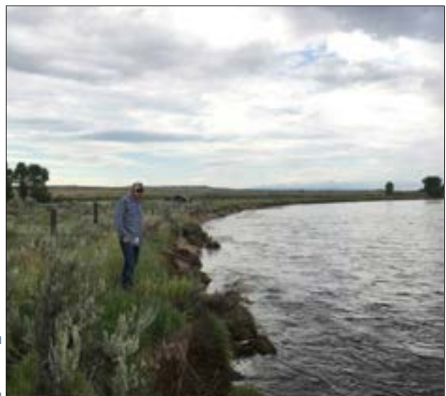
Figure 155. Landowner on the Lower New Fork standing on an eroding bank slated for repair.
