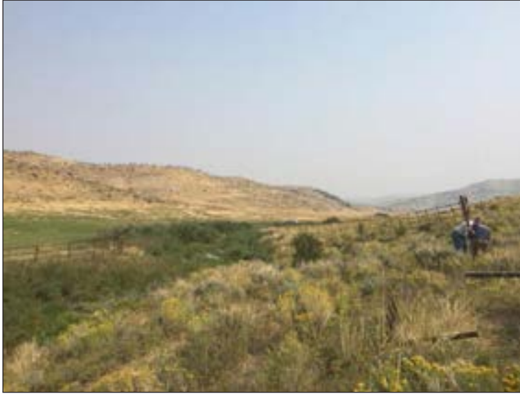
Figure 61. Steel jack fence installation along Trout Creek to protect the riparian corridor. Photo credit Trout Unlimited.
